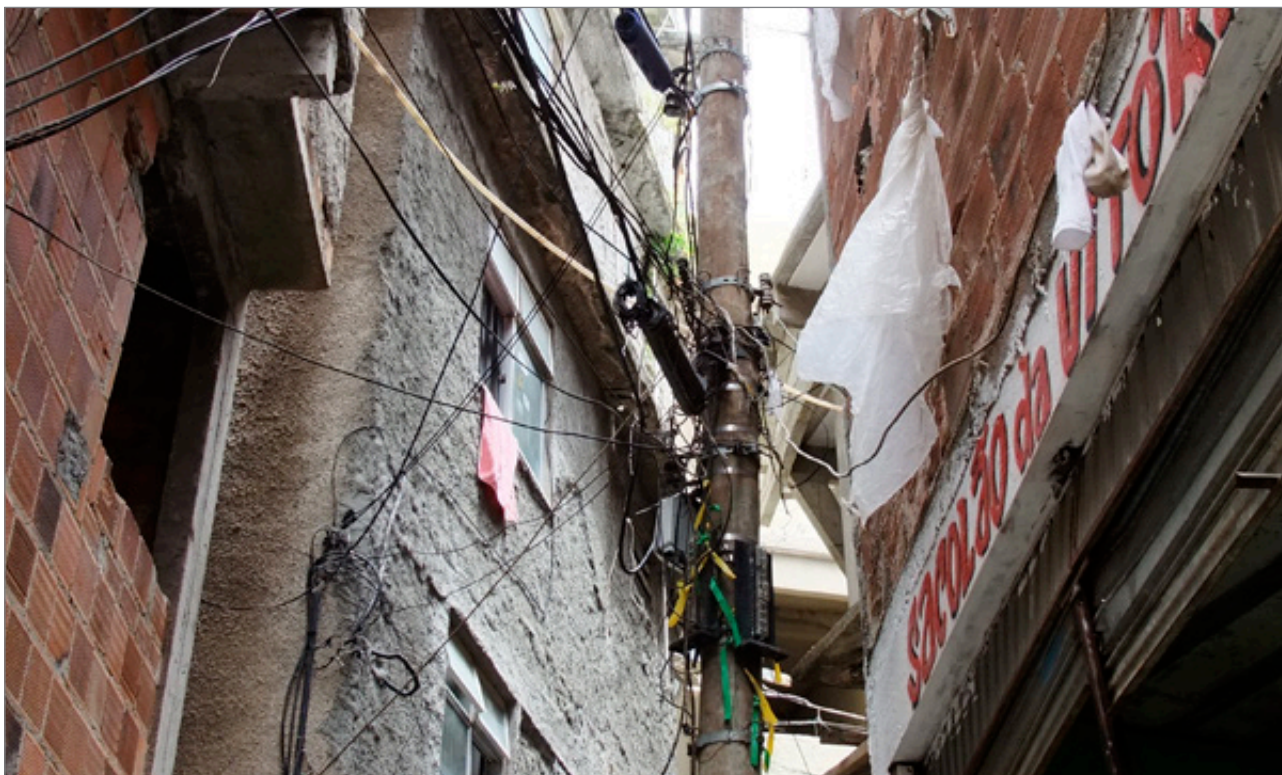
Phone and electricity cables in a lower-income community in Rio.
